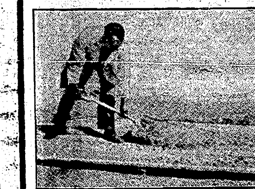
Clean sand is also measured and spread uniformly over the coarse aggregate as shown in the above illustration.
